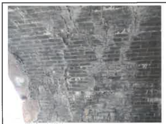
FIGURE 2 - EXTENSIVE CIRCUMFERENTIAL CRACKING WITH LEACHING
