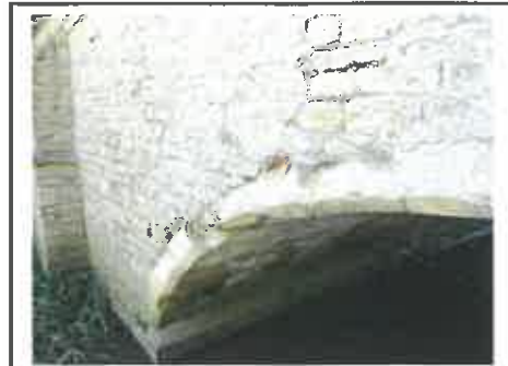
FIGURE 8 – CRACKING AND DAMAGED STONWORK
