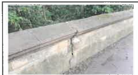
FIGURE 9 – CRACKING AND TWISTING OF PARAPET WALL
