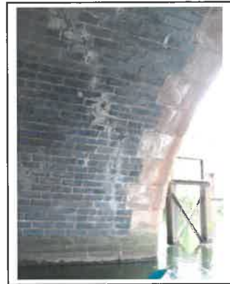
FIGURE 3 - CIRCUMFERENTIAL CRACKING WITH LEACHING
