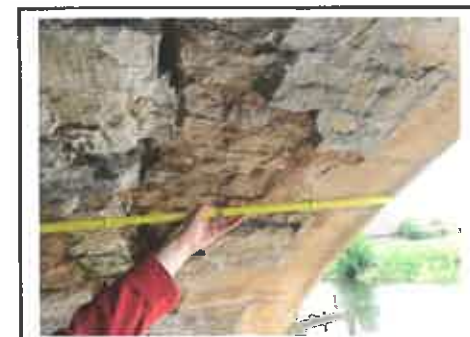
FIGURE 4 - WEATHERED STONE AND CRACK ALONG THE EDGE OF THE VOUSSIORS
