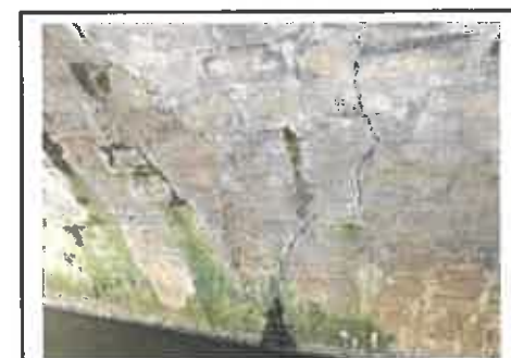
FIGURE 5 - LONGITUDINAL CRACKING IN ARCH
