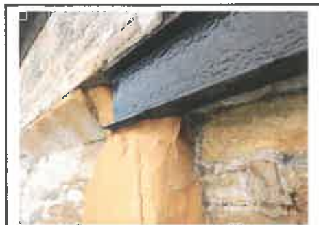
FIGURE 11 – DAMAGE EAST END CORBEL
