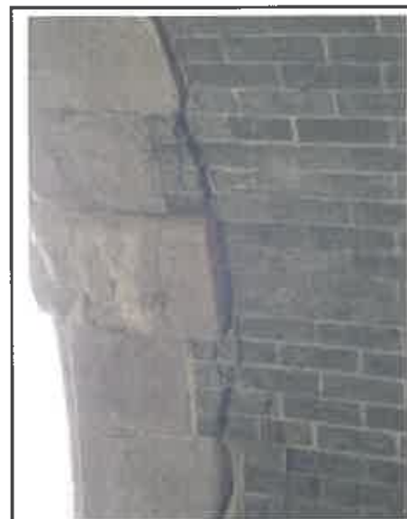
FIGURE 7 - LONGITUDINAL CRACKING BETWEEN VOUSSOIRS AND ARCH
