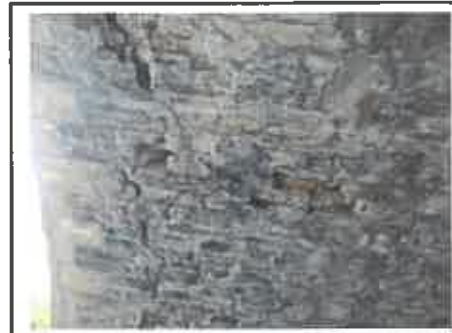
FIGURE 6 - LONGITUDINAL CRACKING AND SPALLING
